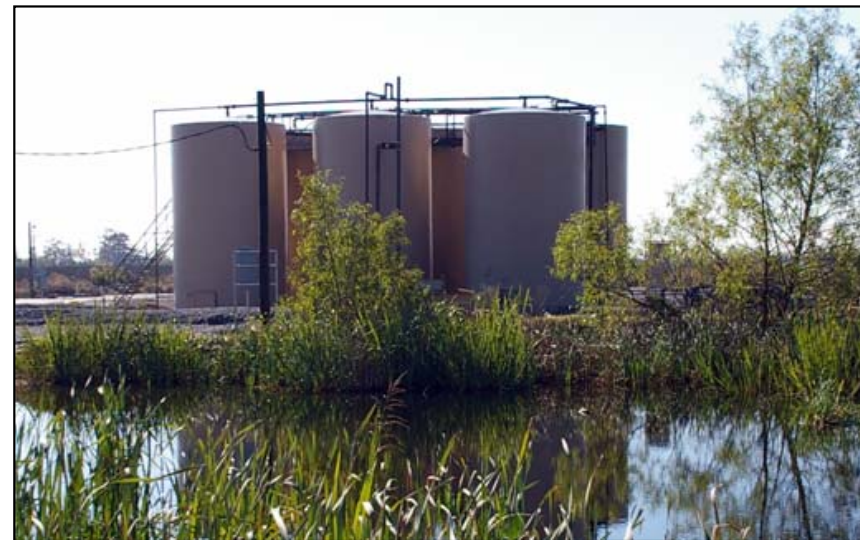
East Chalkley Tank Battery
